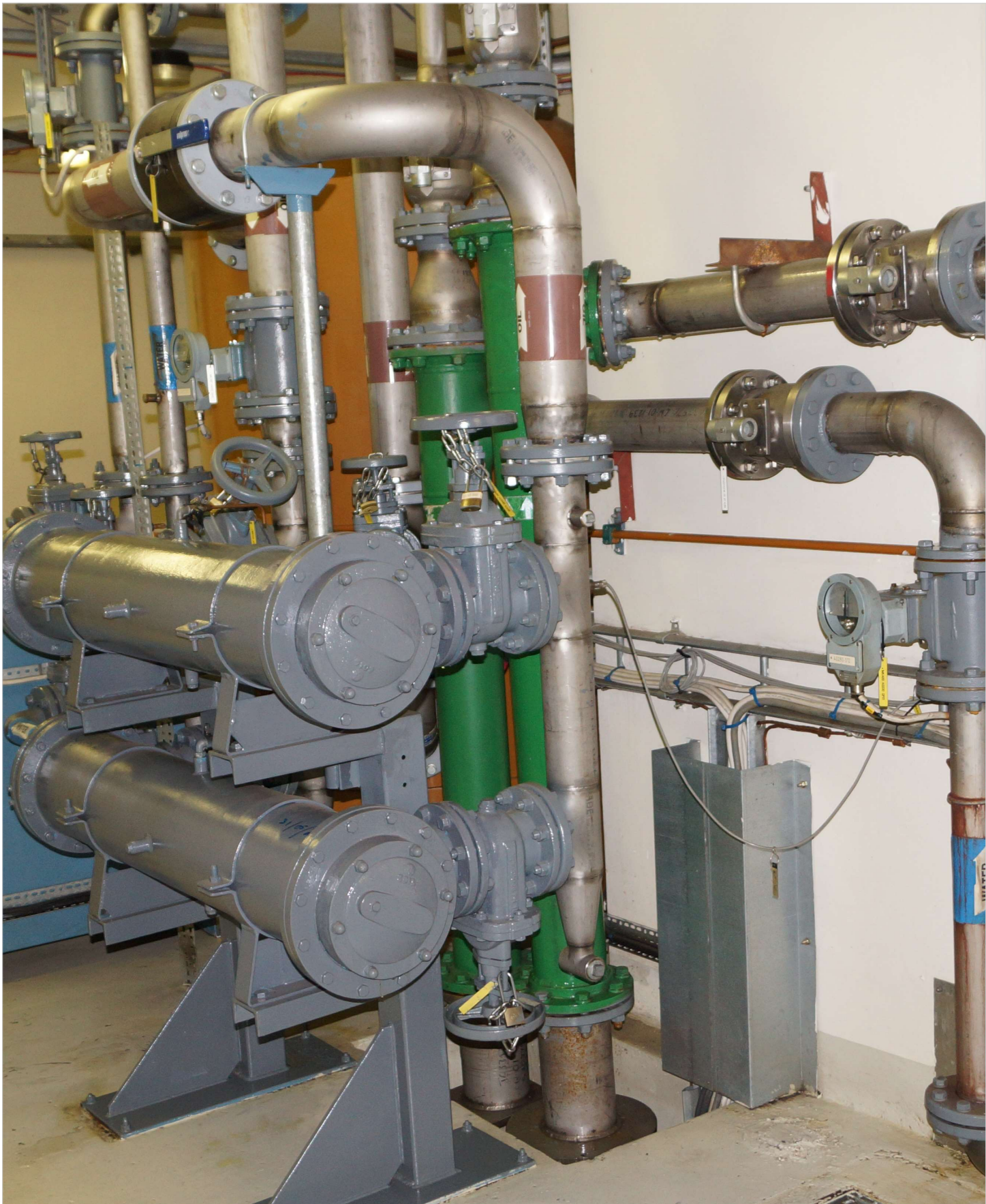
Mechanisms at the 'Muela Hydro-Power Station
