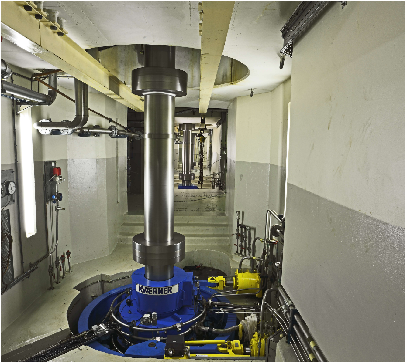
Figure 8: Turbines at 'Muela Hydro Power Station
