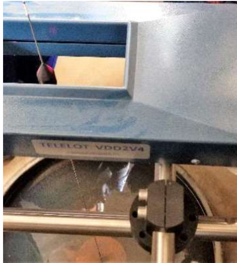
Figure 3: Photo of recently installed automatic pendulum recording station
