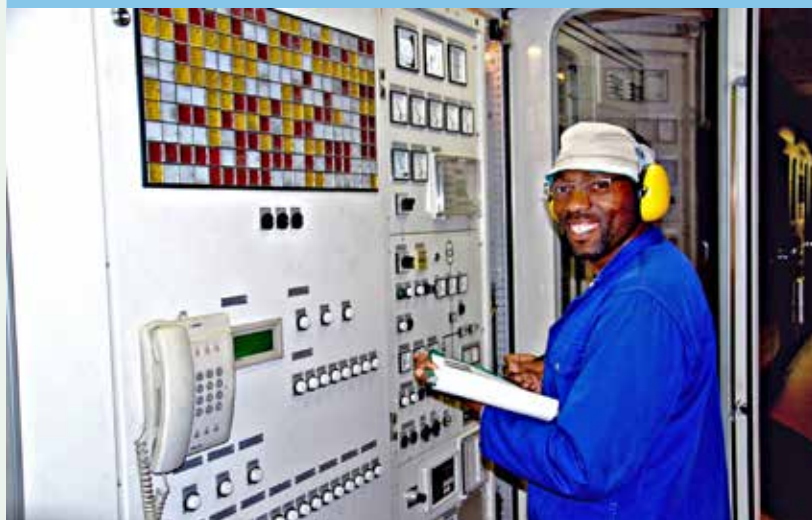
A technician working in the control room at the hydropower station
