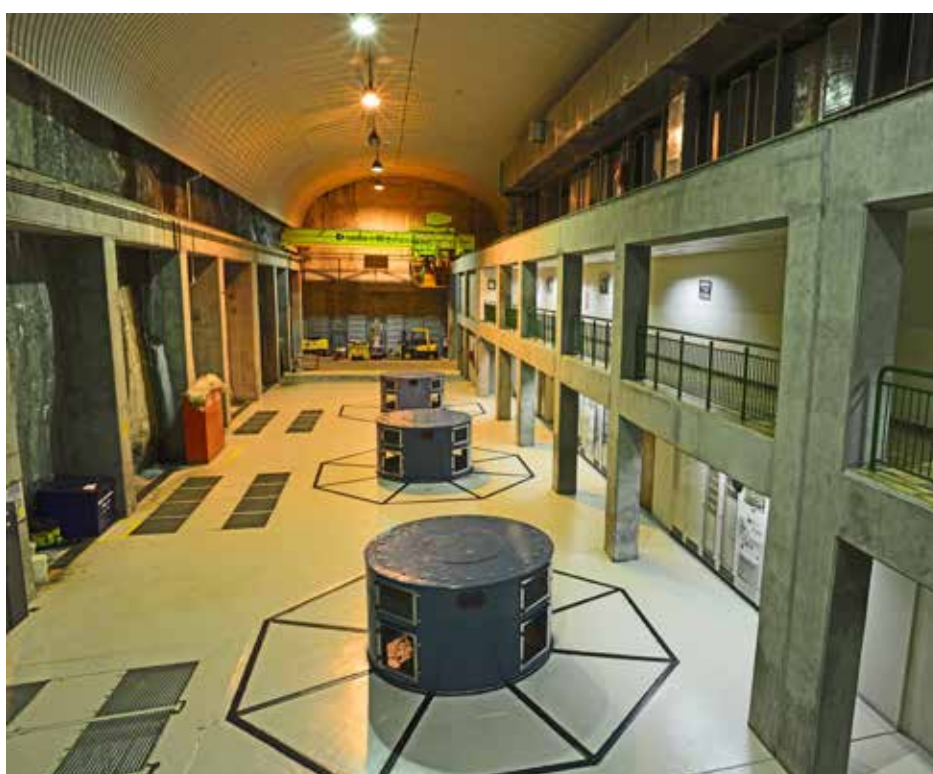
'Muela Hydro Power Station
