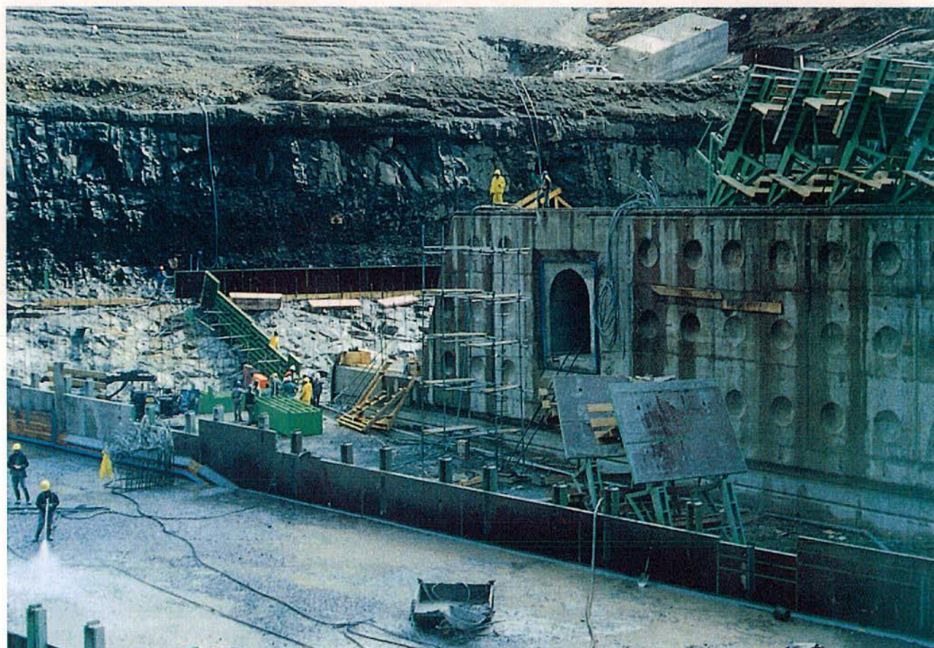
Concrete pouring into the foundations of a double curvature arch dam – Katse
